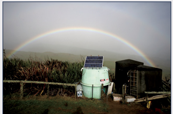
A hilltop wind site with electrolyser hut.
